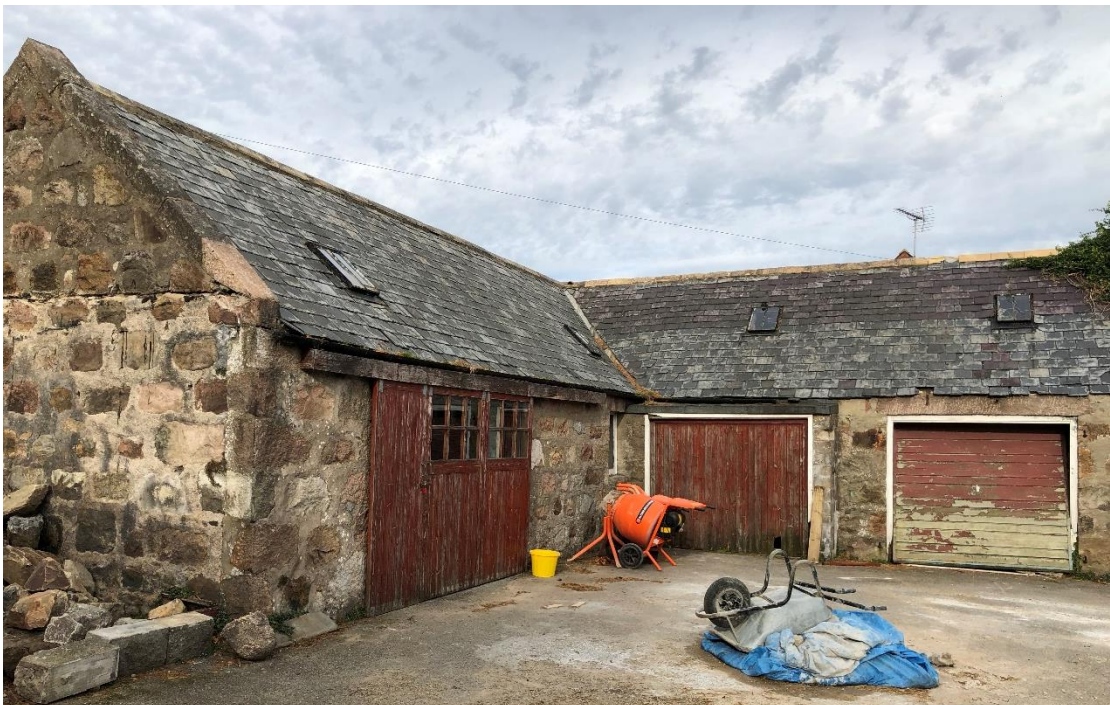
3.08 The steading itself is of low architectural quality. There is very little in the way of foundation. Successive alterations made prior to our clients ownership have led to defects which over time have contributed to overall degeneration of the building fabric.
